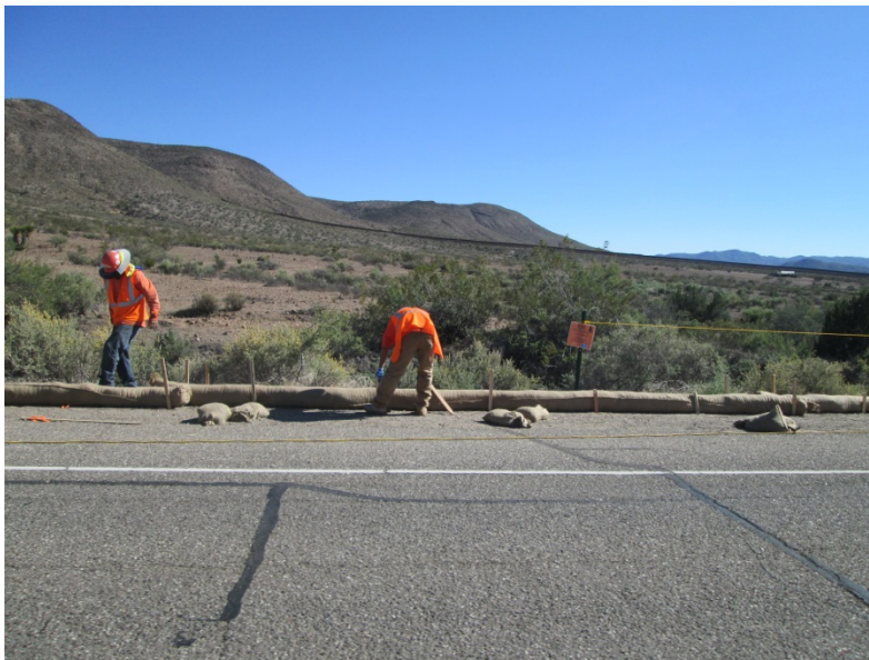
Photo 4: In accordance with the Storm Water Pollution Prevention Plan (SWPPP) (Mitigation Measures HYD-1), straw wattles are placed along the limits of work prior to construction activities being completed along Old Highway 80.
