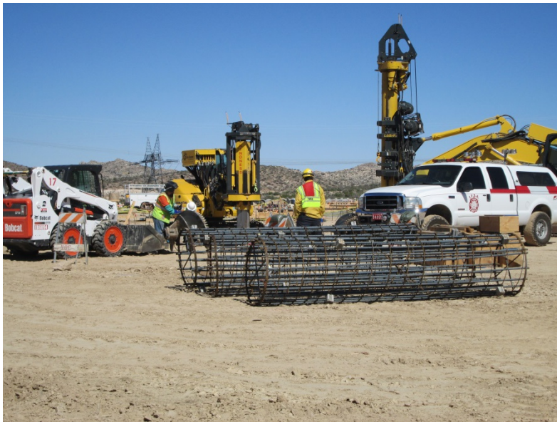
Photo 6: In accordance with the Construction Fire Prevention Plan (Mitigation Measure FF-1), a fire watch oversees welding activities at the ECO substation pad to ensure required fire tools and equipment are on site and that a Hot Work Permit has been obtained as described in NFPA 51B.
