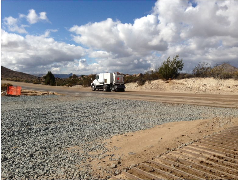
Photo 5: In accordance with the Dust Control Plan (Mitigation Measure BIO-4A), a mechanical sweeper cleans visible soil material along Old Highway 80 at the point of ingress/egress to the ECO substation.
