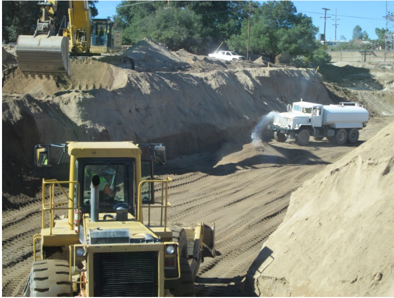
Photo 1: In accordance with the Dust Control Plan (Mitigation Measure BIO-4A), water trucks are utilized to minimize fugitive dust emissions during earthwork activities at the Boulevard Substation.
