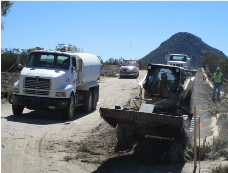
Photo 3: Construction crews complete vegetation removal along the 138 kV Underground Transmission Line from the Boulevard Substation to the 138 kV Overhead Transmission Line. Archaeological, Native American, and biological monitors were observed present during all ground-disturbing activities in accordance with Mitigation Measure BIO-1c and CUL-1d
